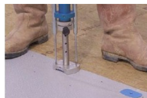
Typical application of a single ply membrane over DuoRock (plain) roofing boards
